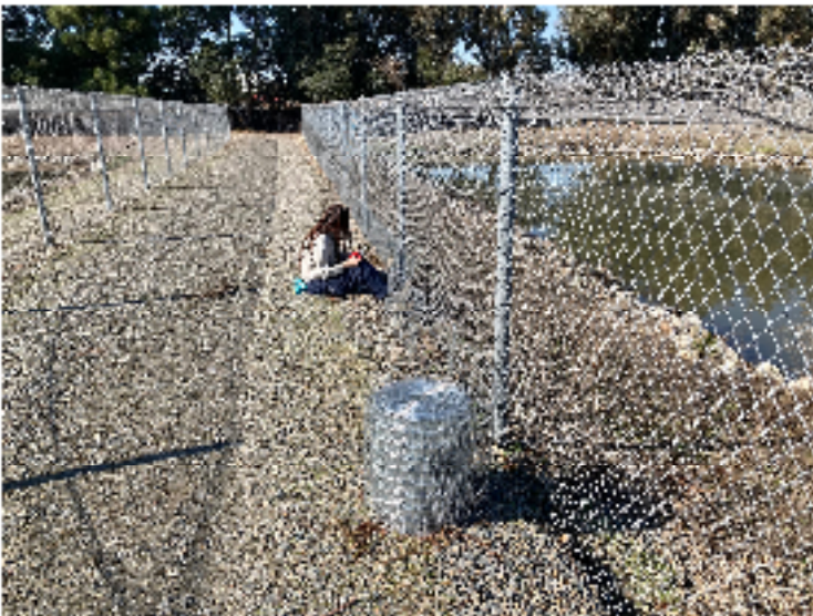
Fence runners being installed to exclude digging predators such as otters, raccoons and turtles.
